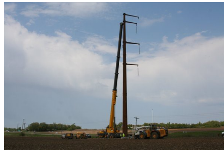
Construction of the HRL transmission project, part of the larger CapX2020 package of projects | Courtesy of CapX2020
